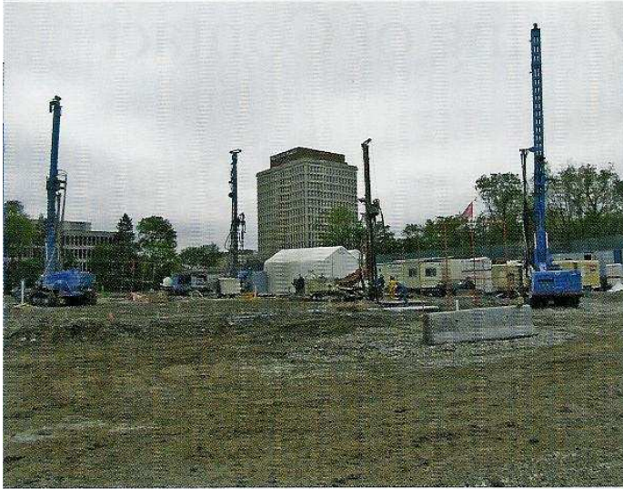
Figure 2. Production oriented drill rigs during drilling of grout holes (courtesy of Layne GeoConstruction).
